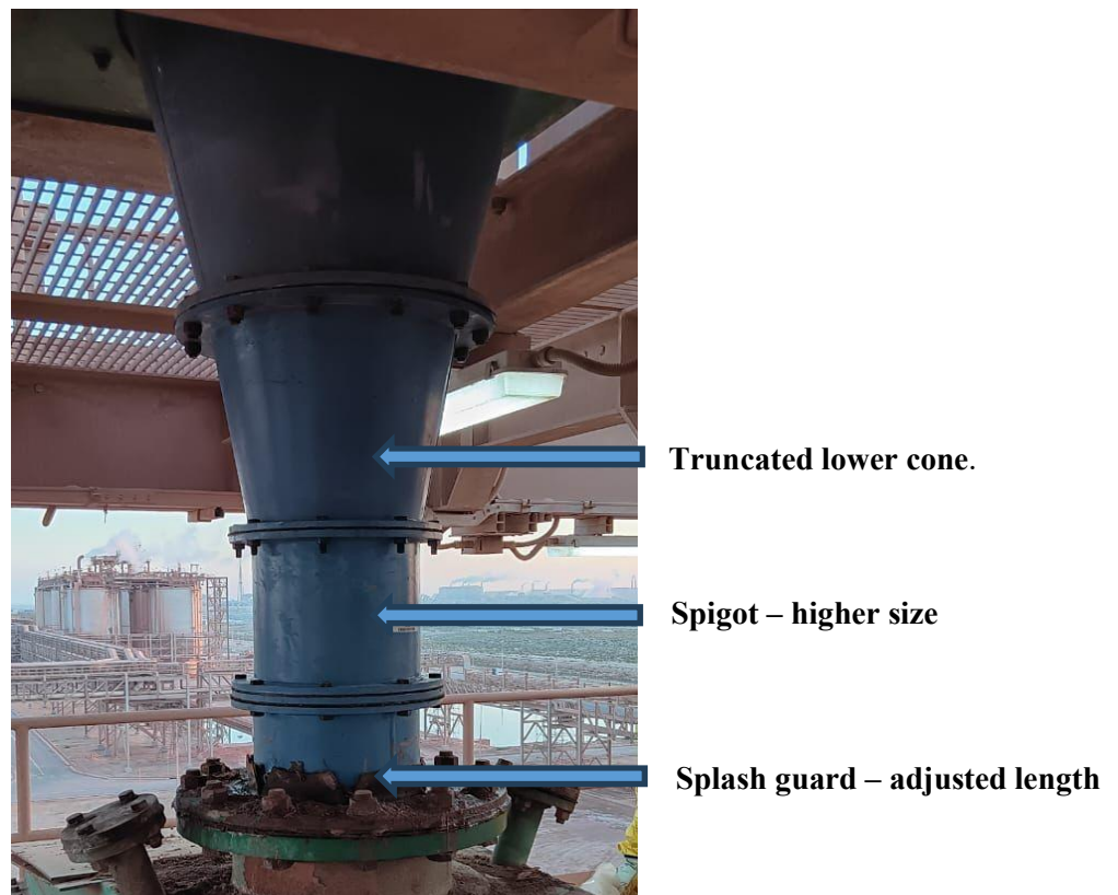
Figure 1. Picture of installed cyclone
